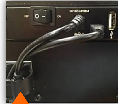
Complete Installation Reference
